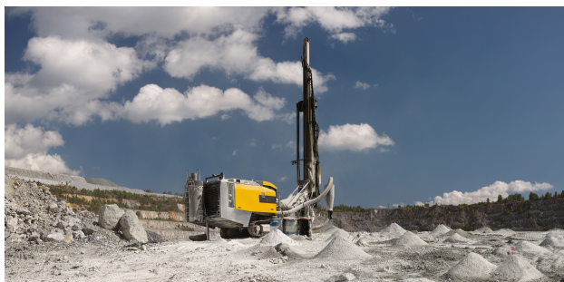
(a) Autonomous open-pit mining: Phase 1 of “drill and blast” method [c5] (source: [29])
